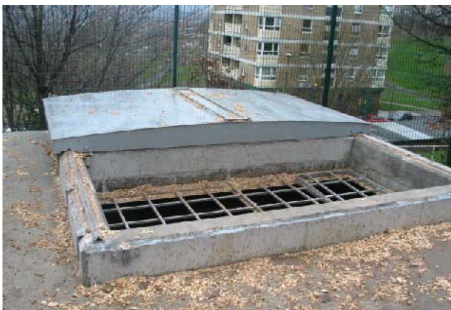
Manual push-back bunker lid awaiting a fuel delivery
